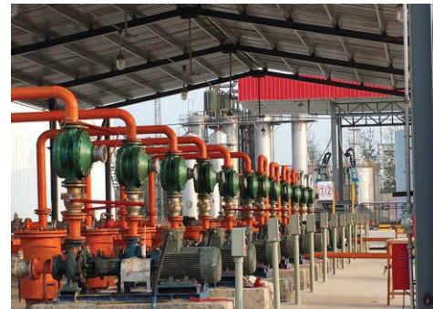
Oval gear flowmeter in petrochemical industry
