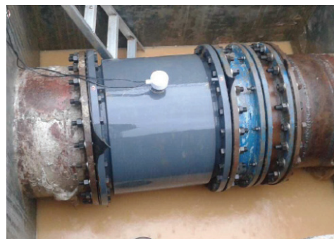
Magnetic flowmeter in under well field
