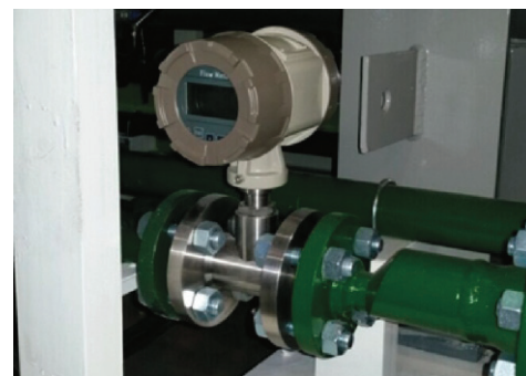
Liquid turbine flowmeter in water supply plant
