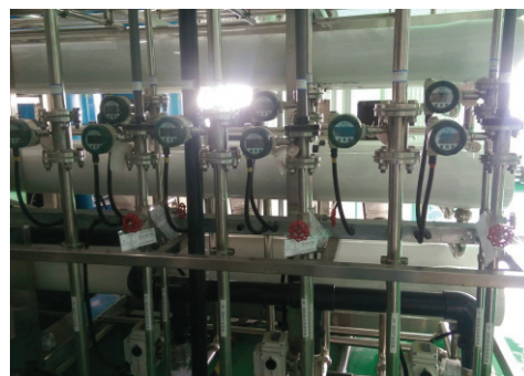
Turbine flowmeter in water supply field
